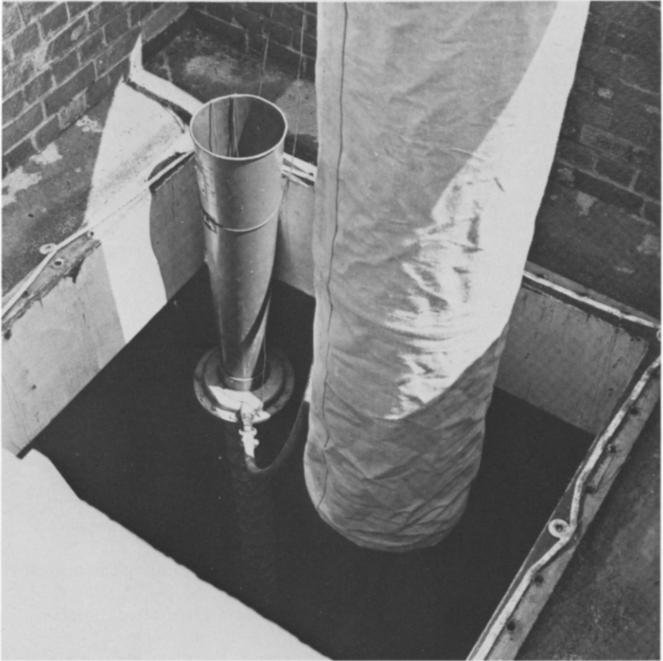
Fig. 2. Compressed air operated venturi air mover (to the left of wind sail air scoop tube).
